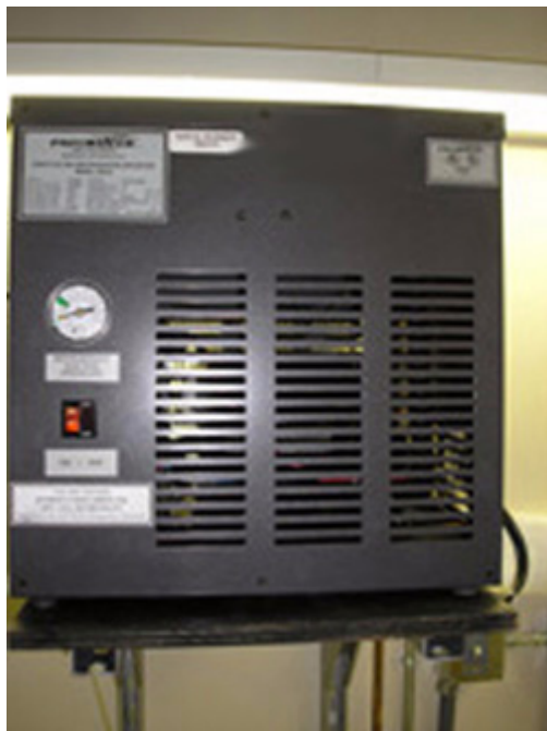
Figure 2-9: Two examples of an air dryer mounted in the Mechanical Room.
