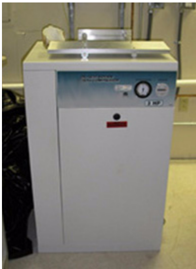
Figure 6-4: Example of an air compressor in the Mechanical Room.
