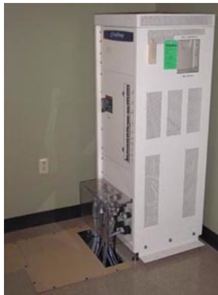
Figure 2-6: PDU in the Equipment Room.
