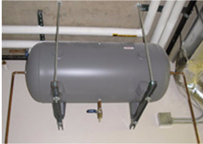
Figure 6-5: Air tank suspended from the ceiling in the Mechanical Room.
