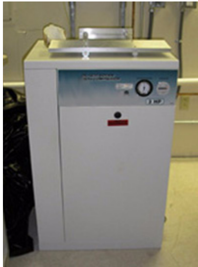
Figure 2-7: Example of an air compressor in the Mechanical Room.
