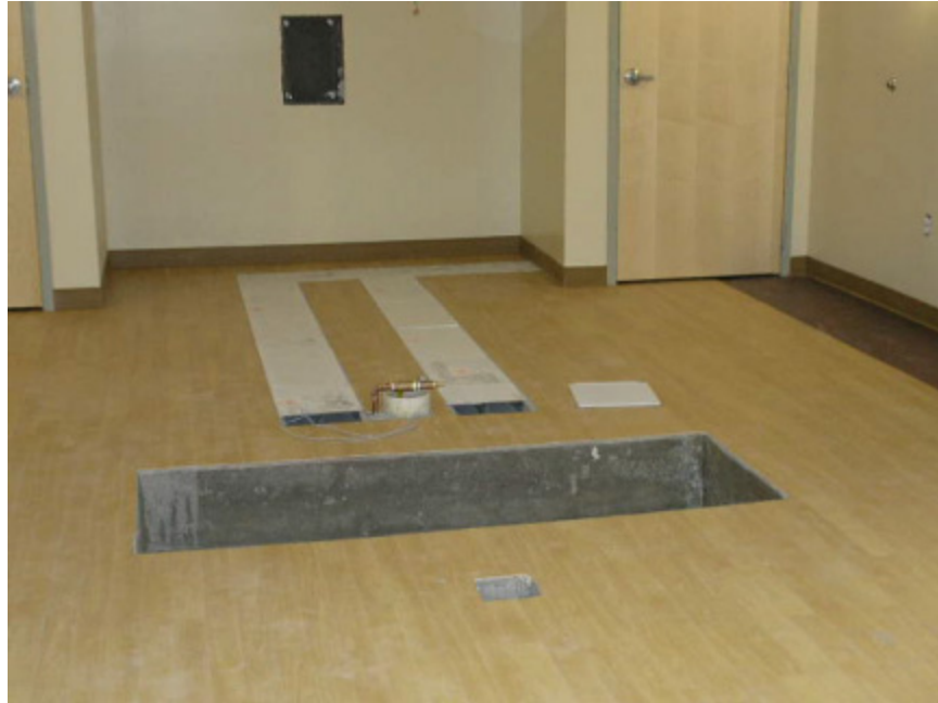
Figure 6-1: Supplemental air duct in back of the gantry pit.
