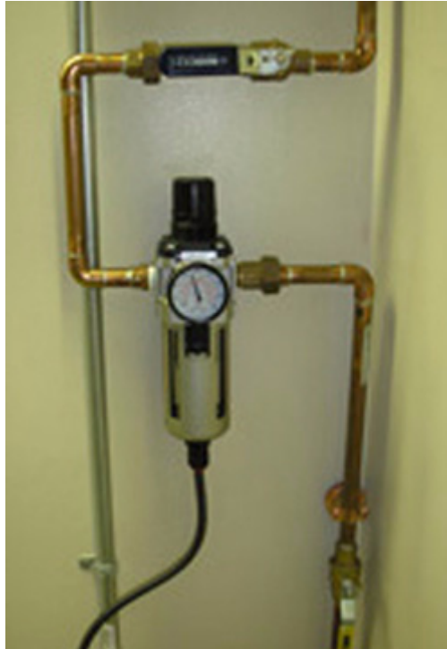
Figure 6-7: Air regulator in the Mechanical Room.
