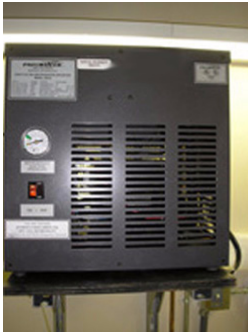
Figure 6-6: Air dryer in the Mechanical Room
