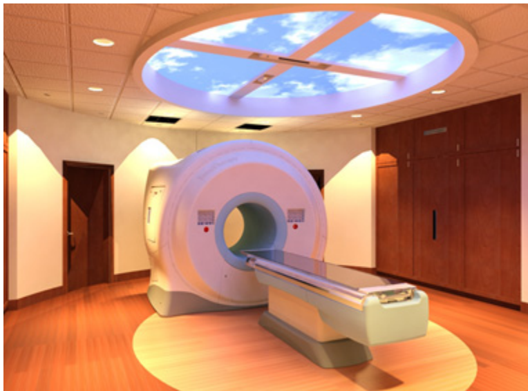
Figure 2-1: TomoTherapy treatment system components in the Treatment Vault (PDU not shown).
