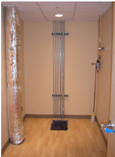
Figure 5-4: Signal cables routed through conduit to the PDU junction box.
