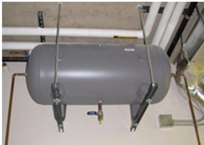
Figure 2-8: Air tank suspended from the ceiling in the Mechanical Room.
