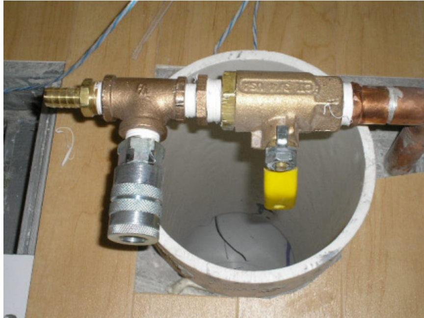
Figure 6-2: Terminated compressed air line with quick-disconnect fitting.
